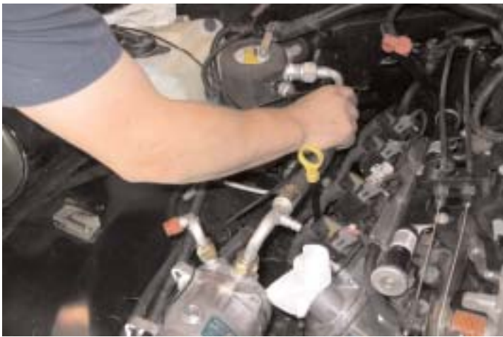
Attaching the new AC line from the 508 compressor to the factory dryer. When installing the AC lines, be sure to coat the threads with refrigerant oil.
